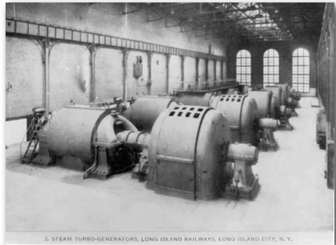
Steam generators, Long Island Railways c.1907
